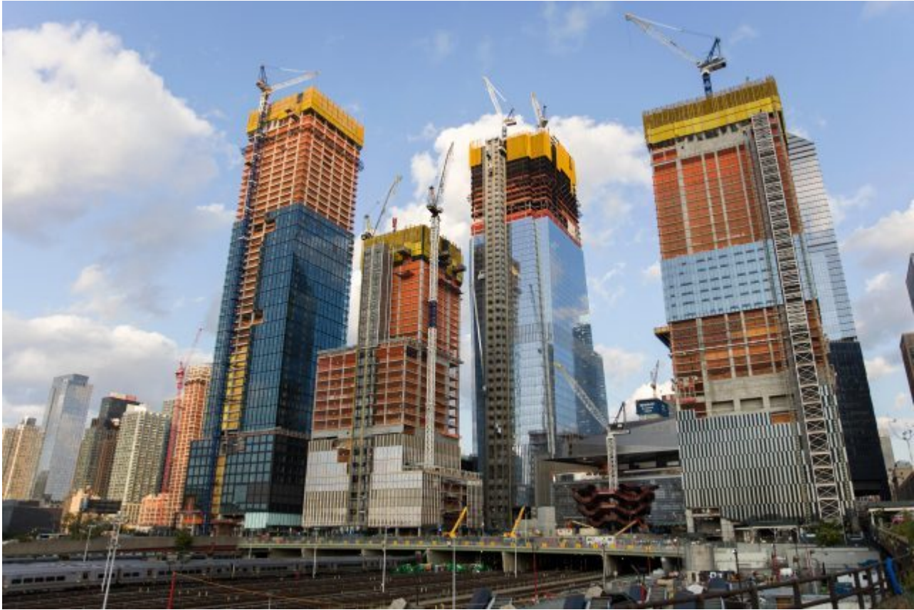
Construction in West Chelsea, New York. Photo credit: Goran Bogicevic/Alamy Stock Photo
